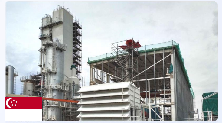
Singapore Jurong Island Air Separation Unit Noisy hood
