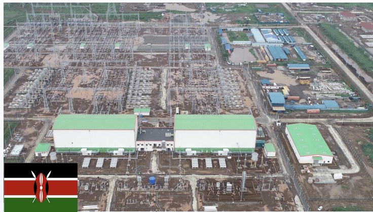
Siemens Kenya high voltage switching station
