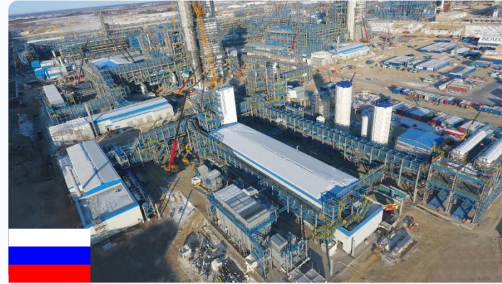
Amur Gas Processing Plant in Russia
